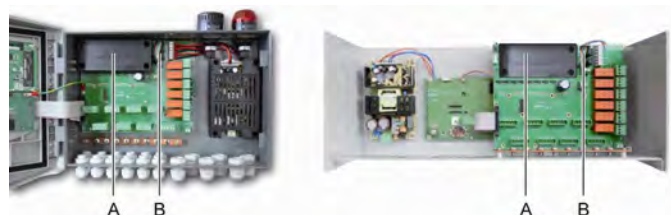
Figure 28: Positioning the battery pack.
